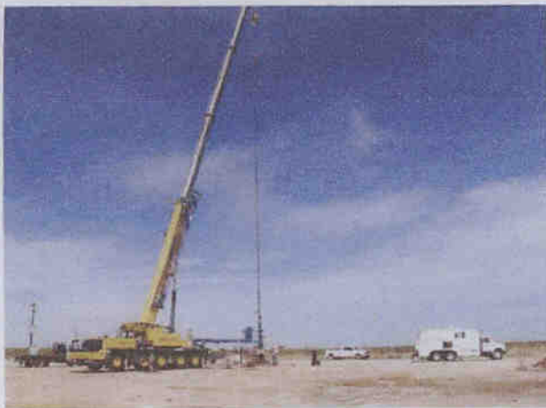
Figure 1. Live well installation of rigless ESP using slickline unit, lubricator and crane (rigless ESP inside lubricator).
